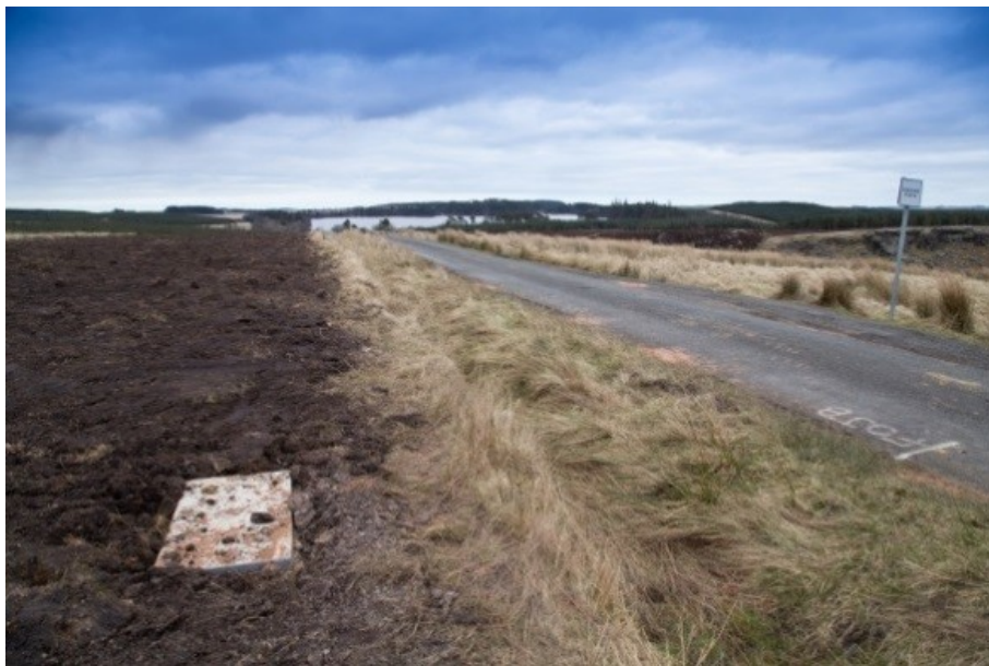
Plate 2 Example below ground link box following reinstatement (Source: Rey Wind Farm, VWPL.)
